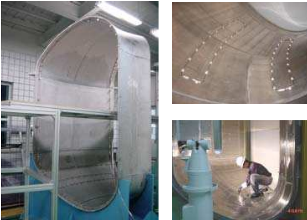
Fig. 4. Installation verification on MDIC.
